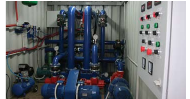
Below: The control room for the new blending plant
